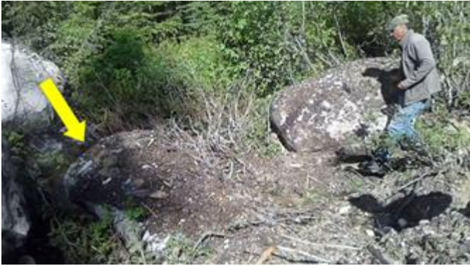
Yellow arrow indicates large culvert that was crushed when boulders (in the pictures) were pushed on top of them.
